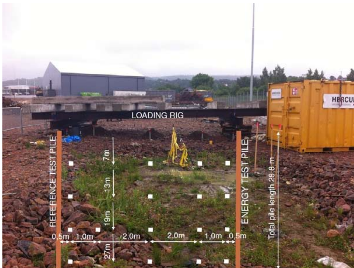
Figure 3. Utby test site. Position of sensors (BAT) in the ground for logging of temperature and pore pressure in the soil.
