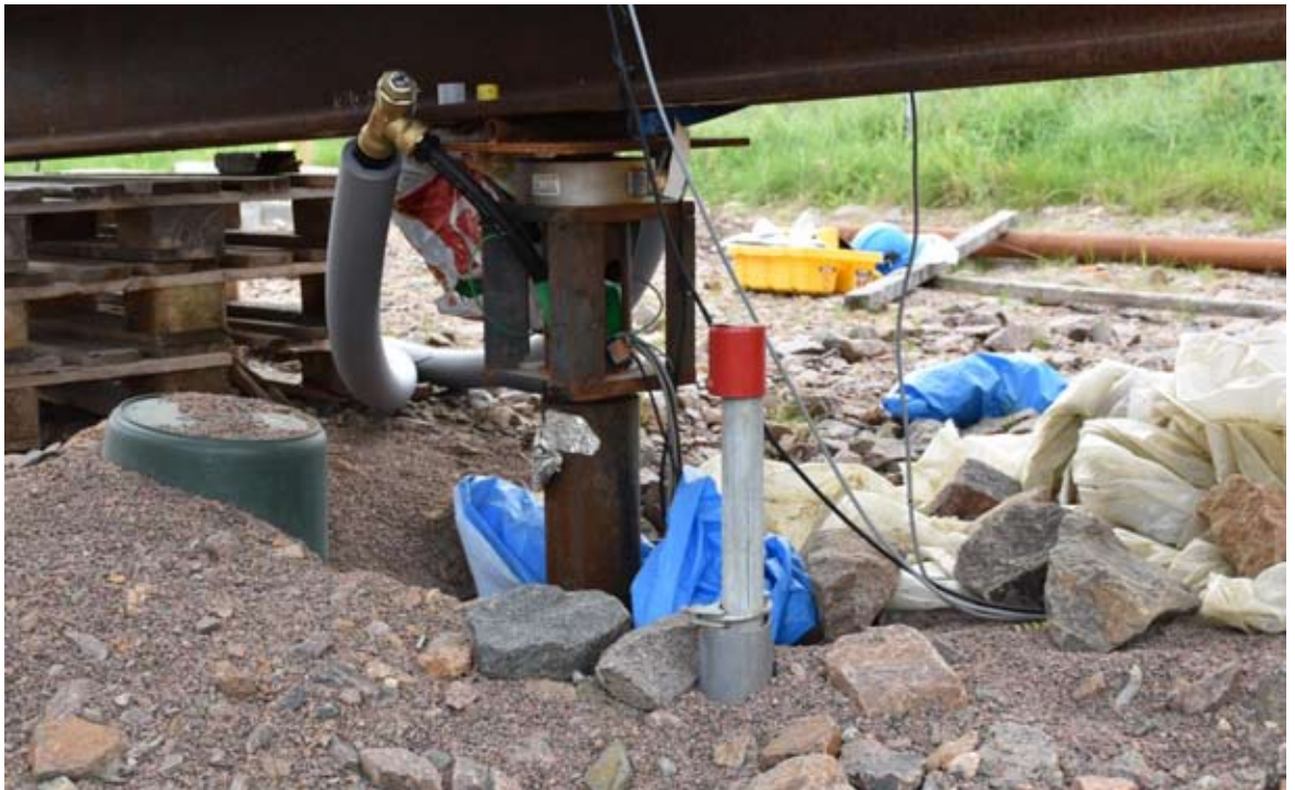
Figure 2. Pile head of the steel thermal pile at Utby with U-tube heat exchanger, fibre optics for distributed temperature sensing, and cables, before final insulation. The pipe with a red cap is the head of a bellow hose used for settlement measurement. Below the bucket to the left is a station of 4 pore pressure and temperature sensors (BAT). A pressure cell for measuring data on static load is placed between the pile head and the steel beam on top.
