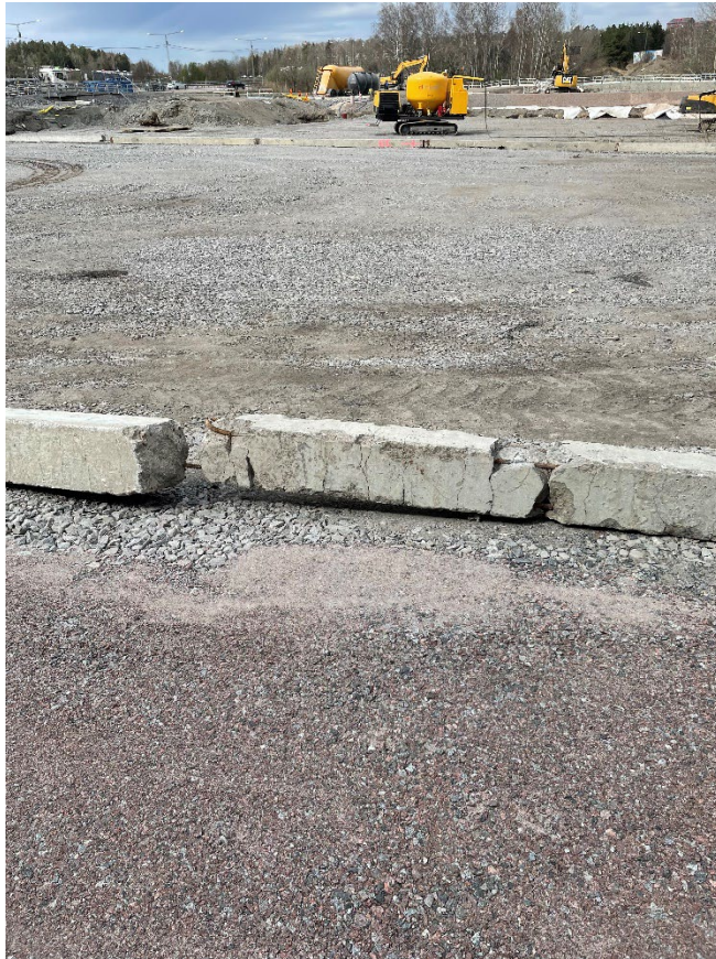
Figur 1. Example of pile refusal for a driven reinforced concrete pile.
