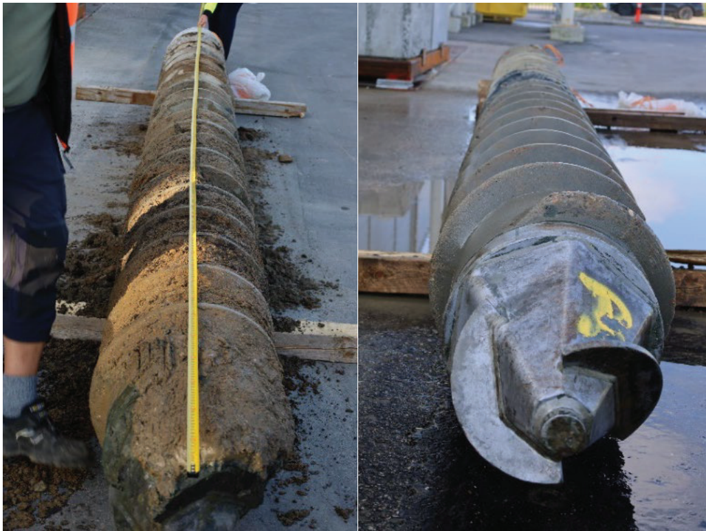
Fig. 7. Inspection of extracted concrete screw pile after installation and static load test
